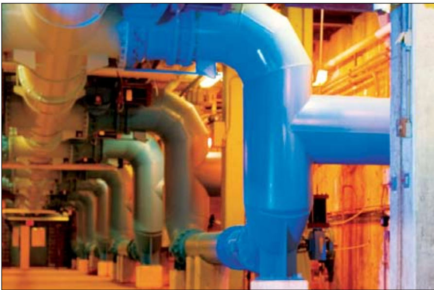
This photo shows the inside of the Dalecarlia Treatment Plant, where approximately 9 billion gallons of Arlington's drinking water is treated each year.
